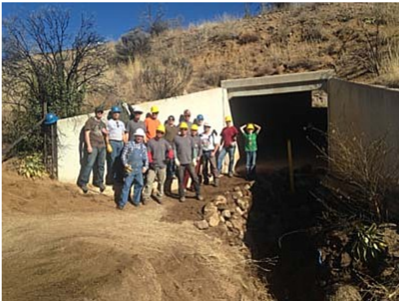
Courtesy PNF/Jason Williams Prescott Trail Riders volunteers show off their hard work to reopen and repair the Box Culvert Trail on the Prescott National Forest west of Prescott.
